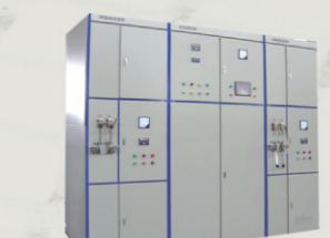
High Voltage Switchgear
